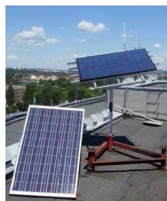
Fig.1. The tracking system and the fixed system with the polycrystalline modules with the power of 210 Wp, micro-inverters and the controller installed on the roof of the Faculty of Electrical Engineering building
