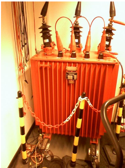
Fig. 81 Distribution transformer HV side 10.5kV, LV voltage side 400 V
