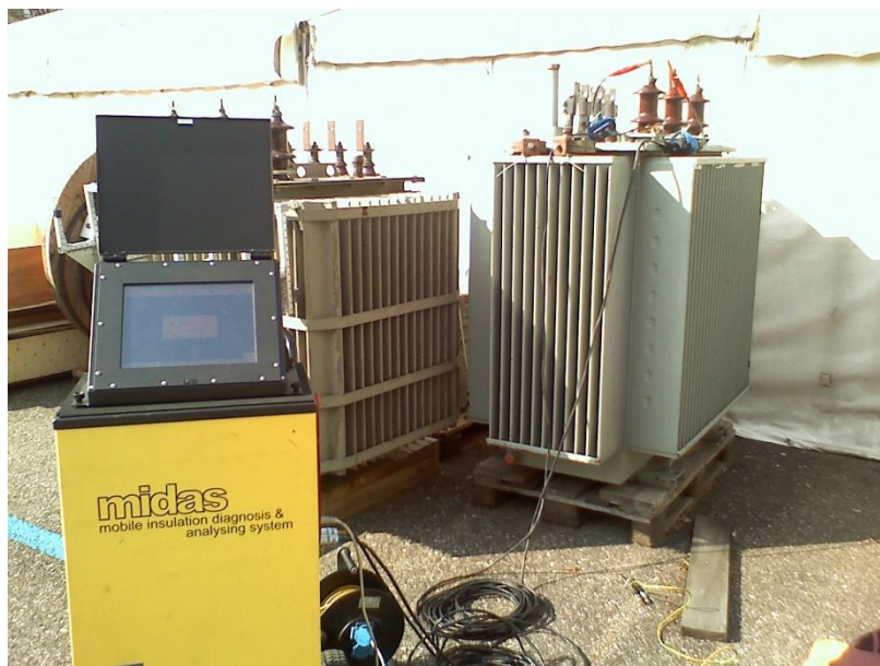
Fig. 84 Distribution transformers Brown Boveri and Breda
