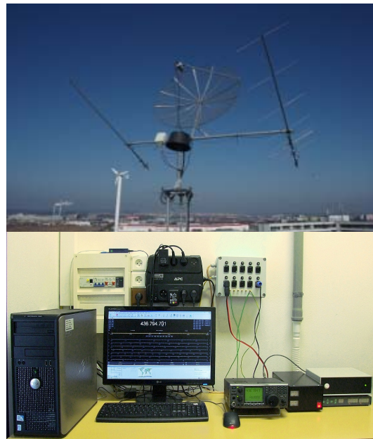
Figure 3. Pilsen ground control station antenna tower and computer control room.
