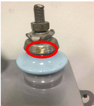
Figure 3. Wear damage power capacitor metal casing
