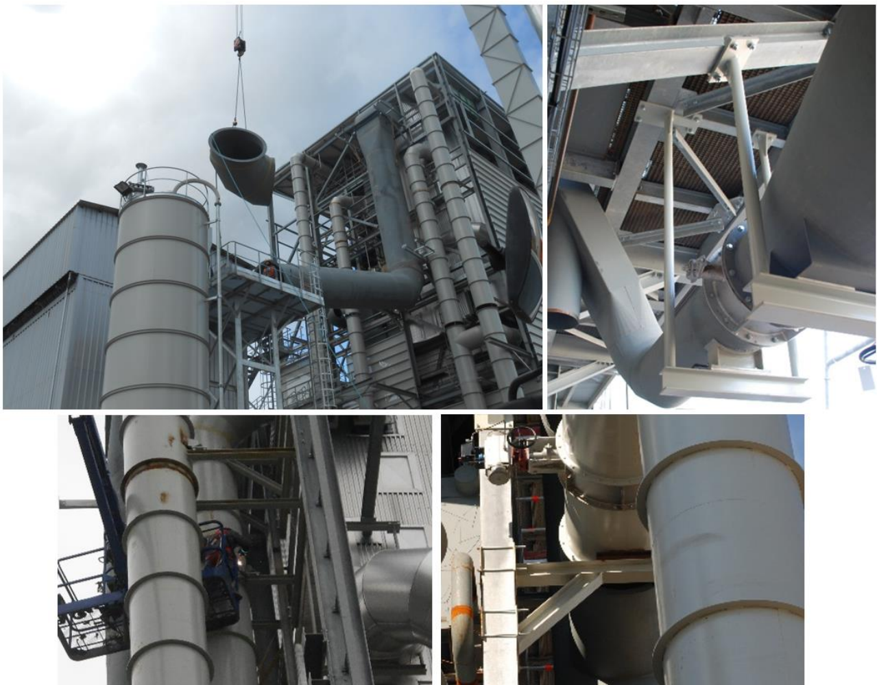
Fig. 12. Photo-documentation from real incinerator construction - detail on selected piping parts and supports
