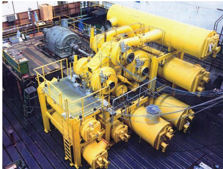
FIGURE 2. Production machine in factories large-scale test bed [10]
