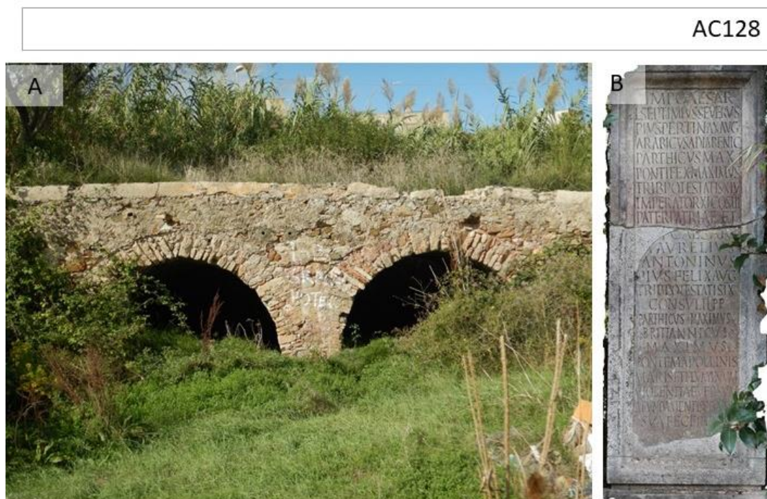
Fig. 147 A: relicts of the bridge AC128 in 2019; B: photogrammetry of the stone Stella.
